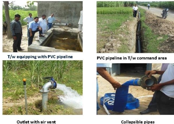
Figure 3.19 Developing water conveyance system in Tube Well command area (UP)
