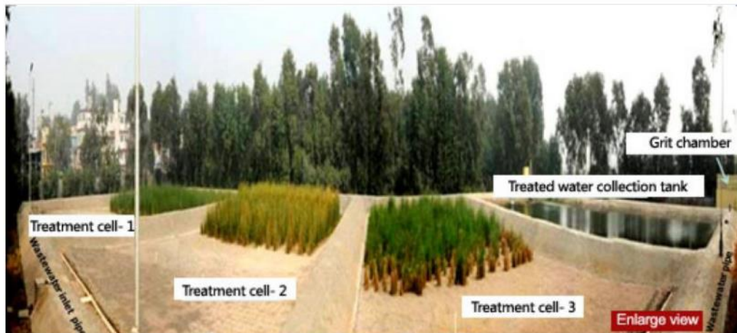
Figure 3.17 Constructed wetland for wastewater treatment at Indian Agriculture Research Institute, Pusa, New Delhi
