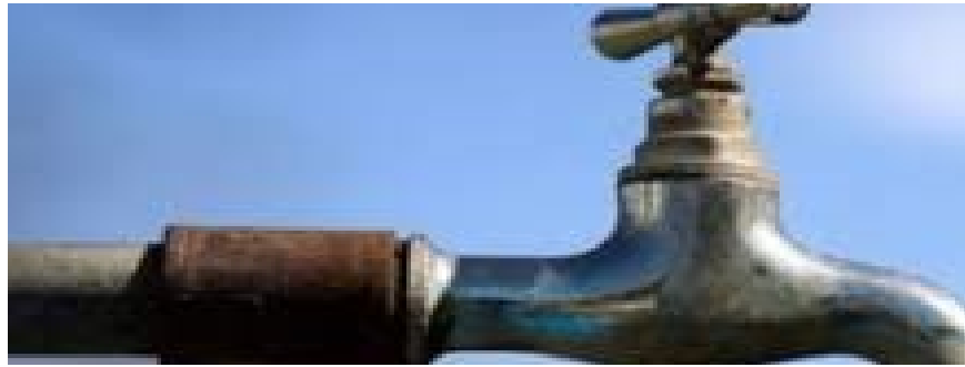
Fig 4.12c: Scene 3- Failure of piped supply of water to villages
