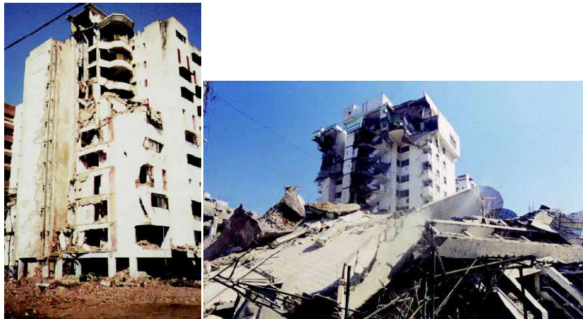
Plate 1: Apartment Building Damaged in Surat and Ahmadabad during the Kutch Earthquake 2004.(Source: NDMA)
