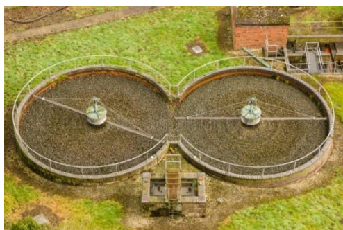
Fig 3.3 Aerial view of Trickling Filter
