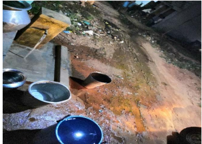
Picture showing how villagers fetching water from taps and they are left unclosed after using thus making surroundings unhygienic
