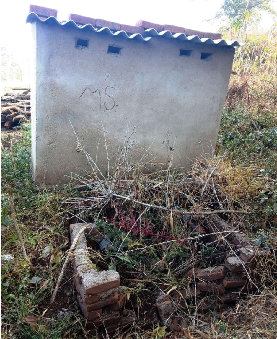
Picture 17: Single pit for two joint toilets shown in Pic. 16 is non-usable condition
