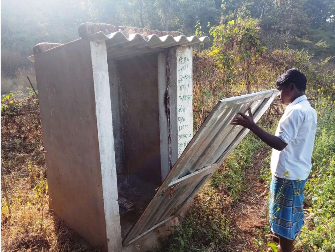
Picture 19: Newly constructed toilet with sub-standard broken door at Upartola, Pharrisemer
