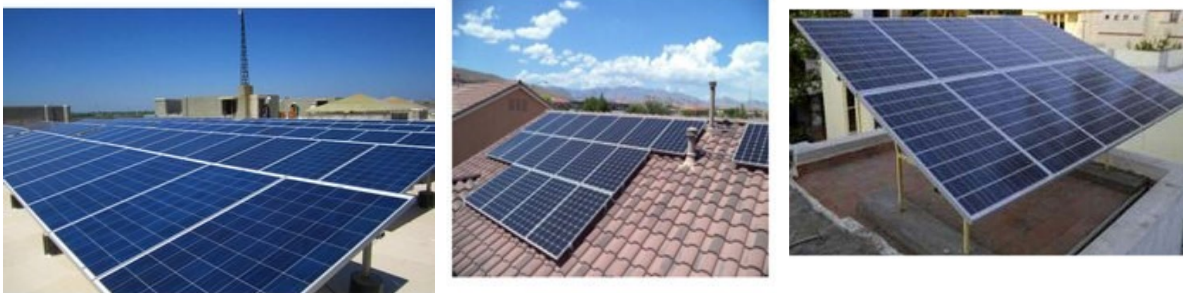
Solar Power Plants
