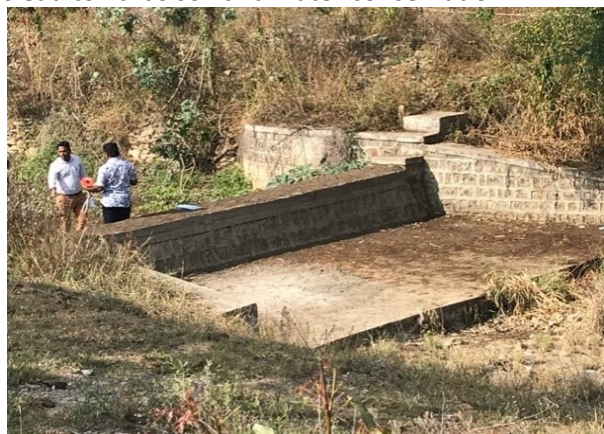
Picture 6.1: Check Dam in Narona (Photographed by Sarvesh Chaturvedi, dated: 21 December 2018)
