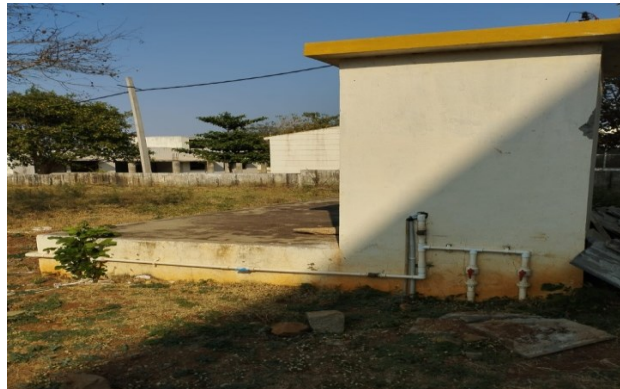
Rain Harvesting Pits
